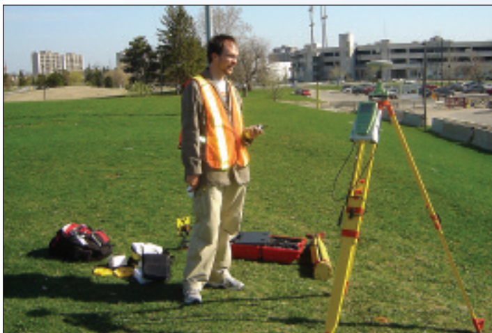
Goran Rauh. Establishing high precision GPS network for monitoring deformations of the Rexall Centre, York University, Keele Campus, August 2007 (Advanced Field Surveys, Photo credit: Prof. Jian-Guo Wang)
